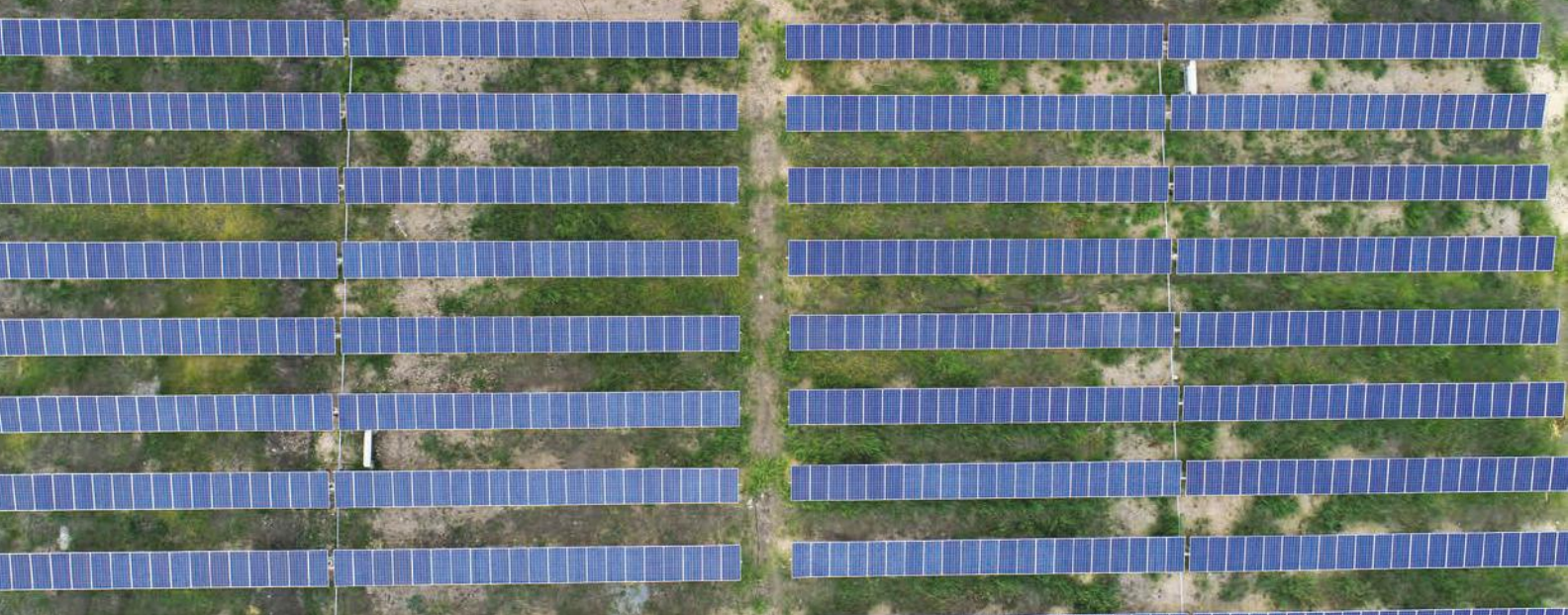
Fig. 1.22. Solar farm near Raichur, Karnataka
