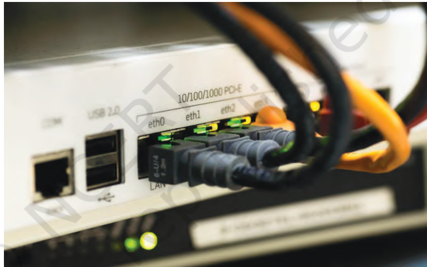
Figure 5.9: Cables connected to a network switch
