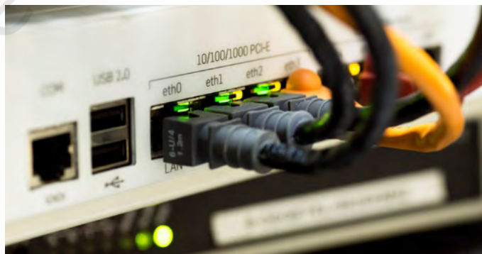
Figure 10.12: Cables connected to a network switch
